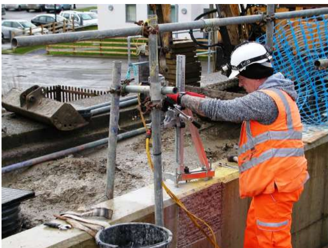
Drilling underway showing clamping bolt in centre of jig base Photo : PR
