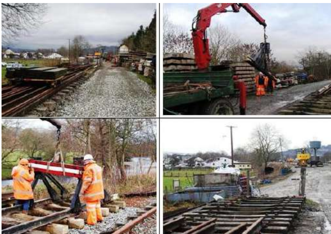
(Clock wise) Buffer stop on main line, Buffer frame on its way to new position, Buffer board being added to frame, Open end looking west Photos : PR
